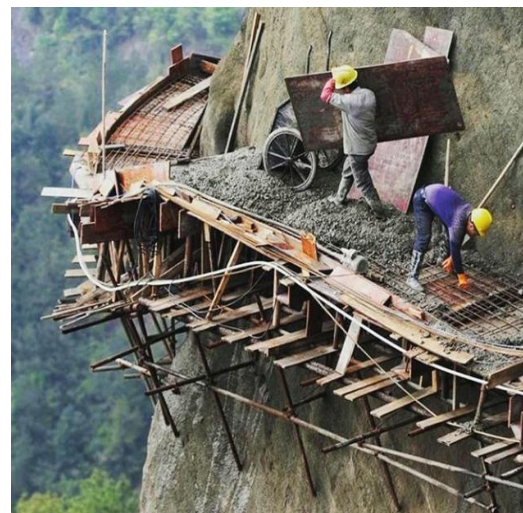
FIGURE 2.3: Difficult and dangerous image of construction industry [50]
