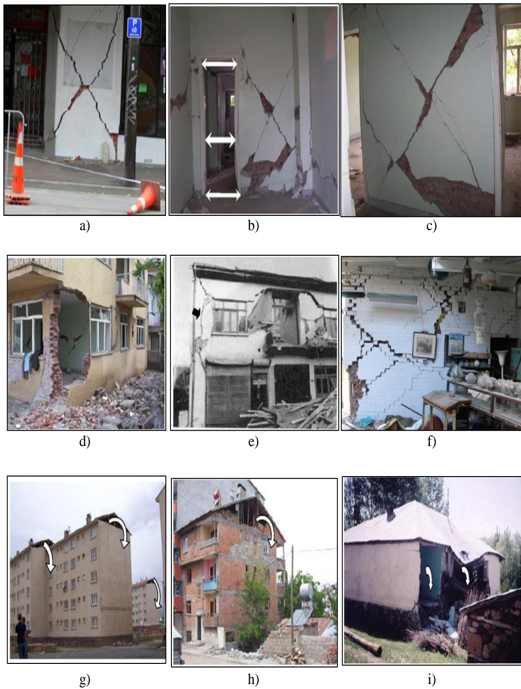
FIGURE 2.2: Masonry Wall Failure; a,b,c) Diagonal Cracks on Wall, d) Separation of Wall, e,f) Vertical and Diagonal Cracks, g,h,i) In-plane Failure [8] and [10].
