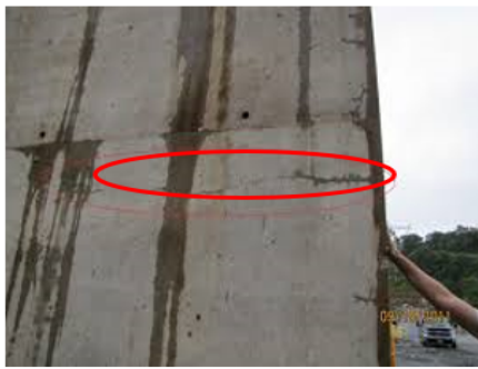
Cracks in Compression Member
