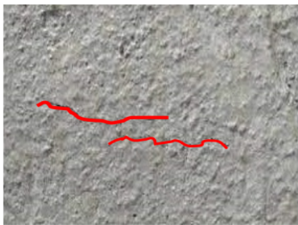
Early Age Micro-Cracking in Slab
