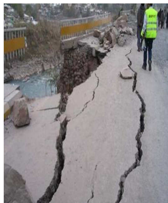
d) Retaining walls collapse along roads
