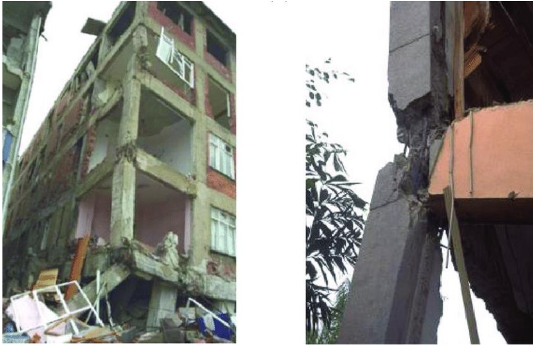
FIGURE 2.1: Structural connections failure
