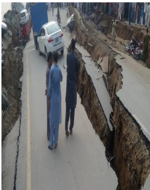
c) Destruction of roads
