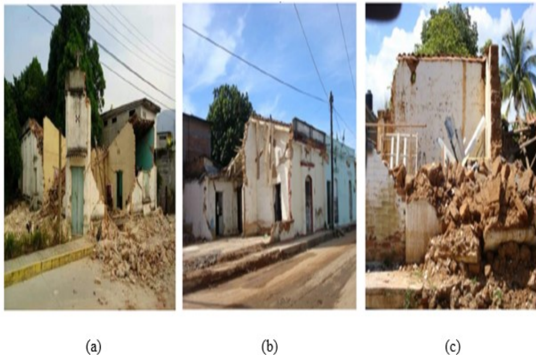
FIGURE 2.1: Diagonal Tension Damage Patterns and Out-of-Plane Wall Collapses in Adobe and Plain Unreinforced Masonry in Housing Structures Located in (a) Pijijiapan,(b) Tonala and (c) Villa Flores Towns of Mexico [14].
