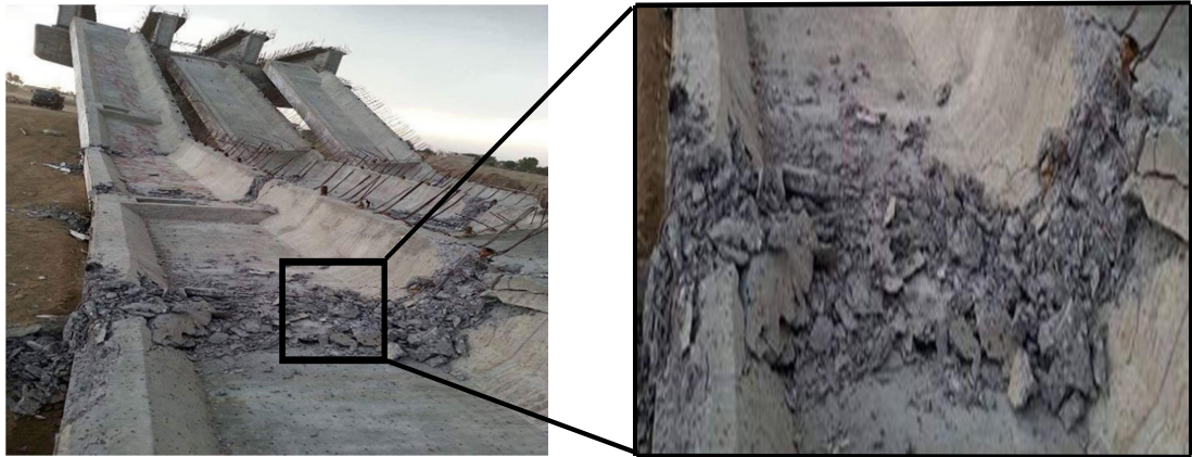
FIGURE 2.1: Failure in concrete bridge girder
