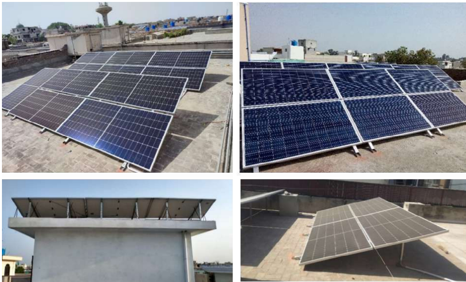
FIGURE 1.13: Roof-Ground Mounts installed at different locations in Pakistan
