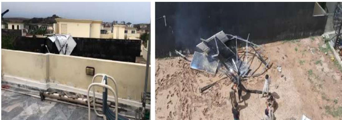
FIGURE 1.15: Damage caused on June 13, 2021, Bahria Enclave, Islamabad
