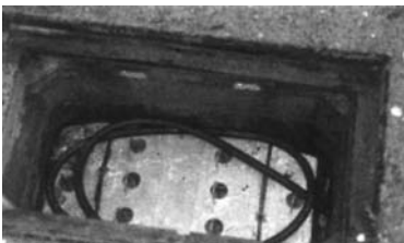
Figure 8.11 Battery in the cable branch box.
