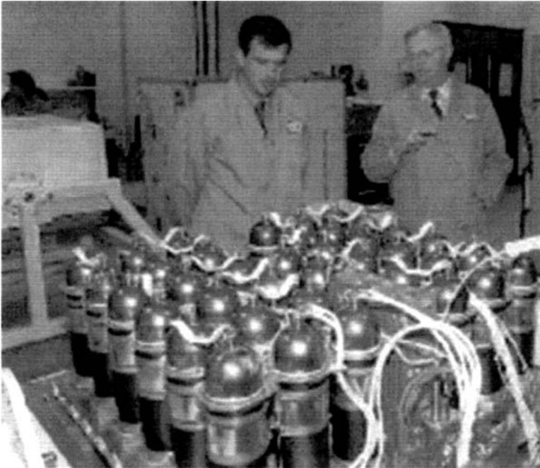
Figure 1.35 A module of 38 cells of a nickel/hydrogen battery that forms one-half of a 76 cell battery ( \approx 100\text{V} ). 24 of such batteries will power the International Space Station (ISS). Cell capacity 85 Ah; stored energy \approx 8\text{ kWh} per battery (from Ref. 61).
