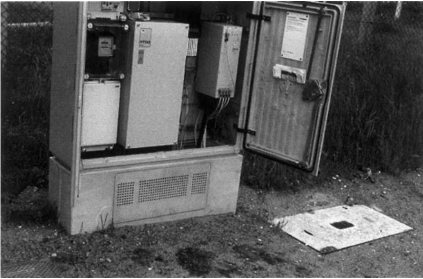
Figure 8.10 KVz cabinet with cable branch boxes.
