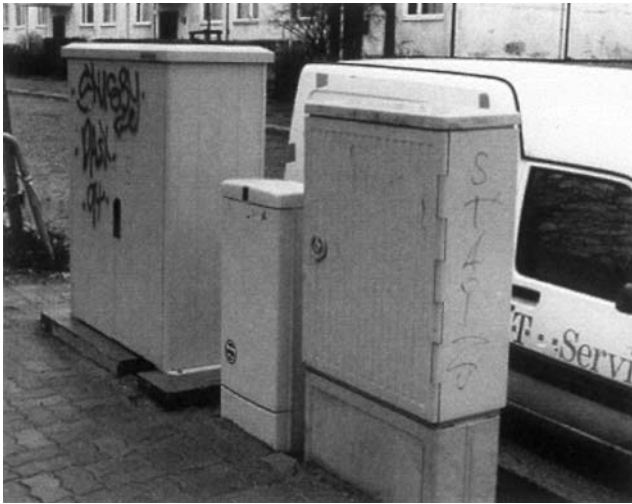
Figure 8.9 KVz cabinet with battery in the pedestal area.
