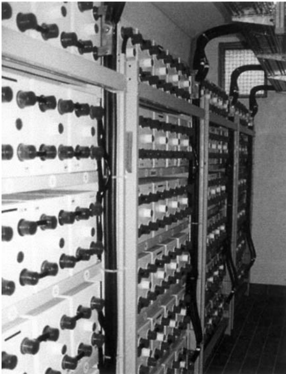
Figure 8.8 Battery area of the MUK.
