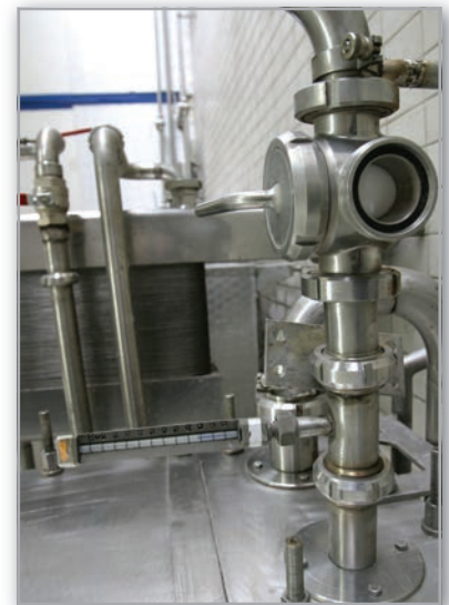
Control Systems (p. 308)
