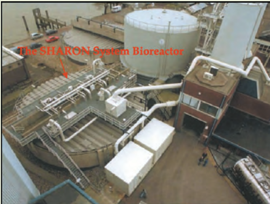
Figure 2 The Sharon (single reactor system for high-rate ammonium removal over nitrite) system bioreactor, Rotterdam, the Netherlands. (Photo courtesy of Grontmij NV, the Netherlands.)
