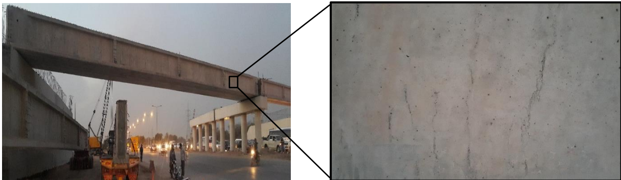
Figure 2-1 Observed EAMC in recently constructed concrete bridge girder
