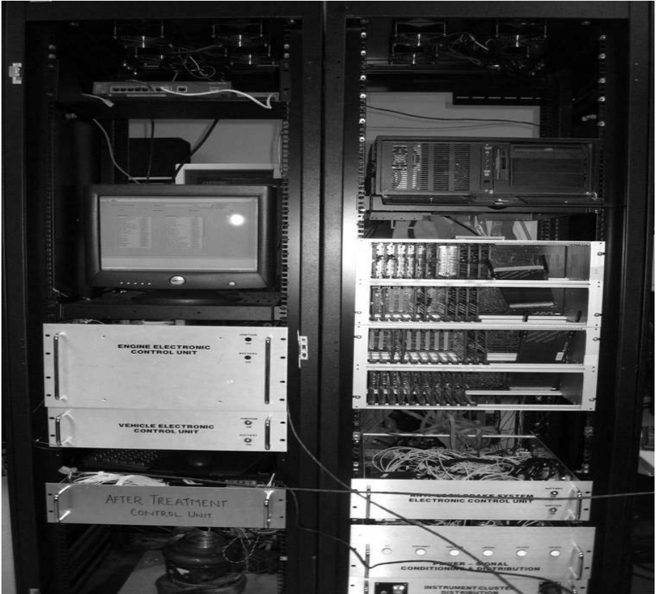
Figure 2.4 The entire vehicle HIL rig, showing the electrical controller unit (ECU) cabinet.
