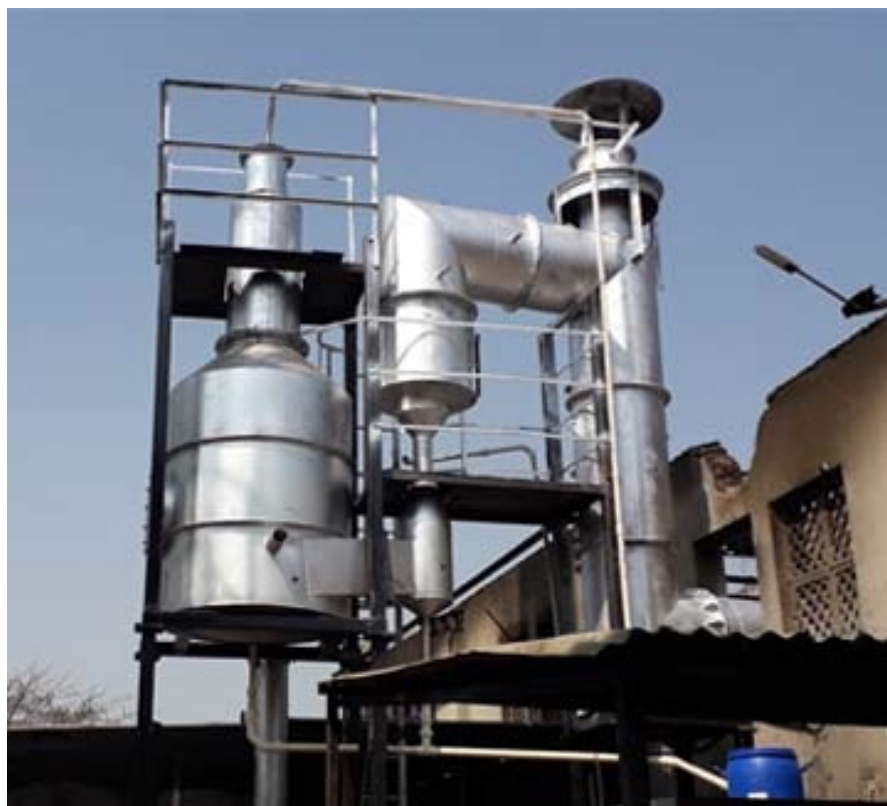
FIGURE 2.2: Incinerator for BMW final treatment (Disposal of BMW)
