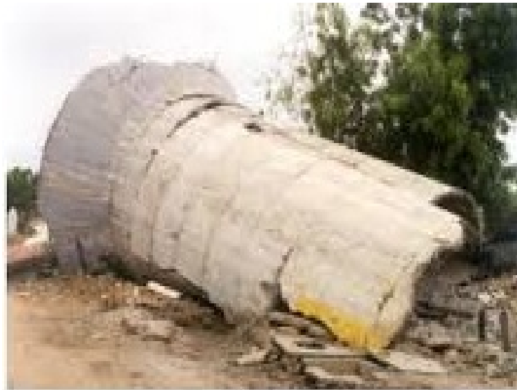
FIGURE 2.1: Damage Mushroom type Elevated water Tank [13]
