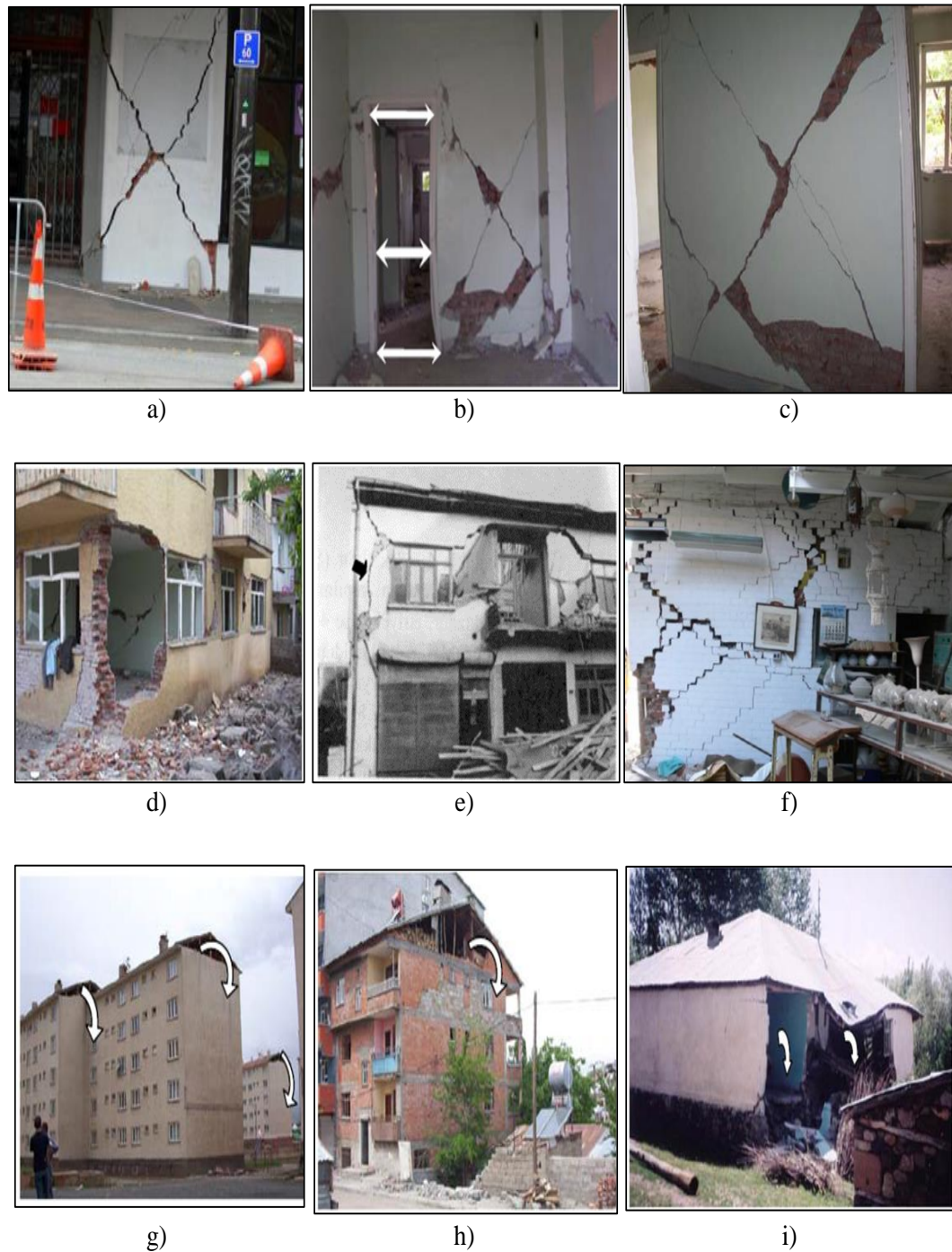
FIGURE 2.2: Masonry Wall Failure; a,b,c) Diagonal Cracks on Wall, d) Separation of Wall, e,f) Vertical and Diagonal Cracks, g,h,i) Out-of-plane Failure [8] and [10].
