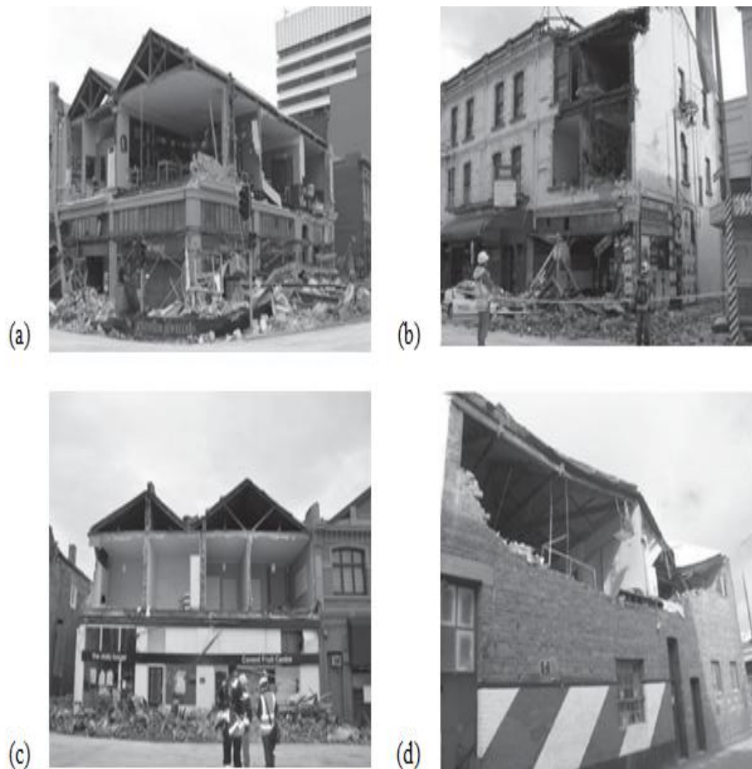
FIGURE 2.1: Masonry wall damages; (a) corner failure; (b) wall collapse; (c) wall collapse at 1st story; and (d) out-of-plane collapse [18]
