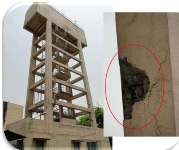
FIGURE 2.2: Cracks located at rectangular OHWT, Dutta et al. (2016).
