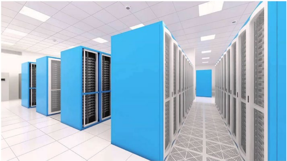
Figure 8-2. Server racks in a datacenter
