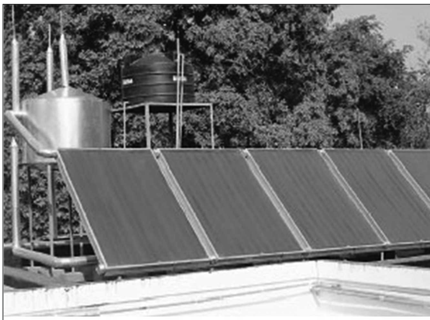
Figure 5.18 Solar water heater
