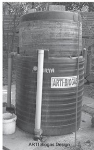
Figure 8.17 ARTI biogas plant
