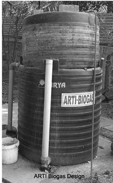
Figure 8.17 ARTI biogas plant
