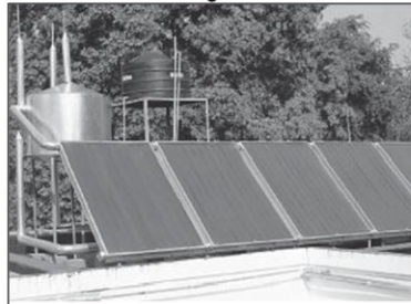
Figure 5.18 Solar water heater
