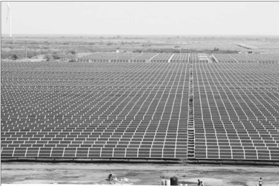
Figure 6.52 A 221 MW Solar Park at Charanka Village, Distt. Patan, Gujarat, India
