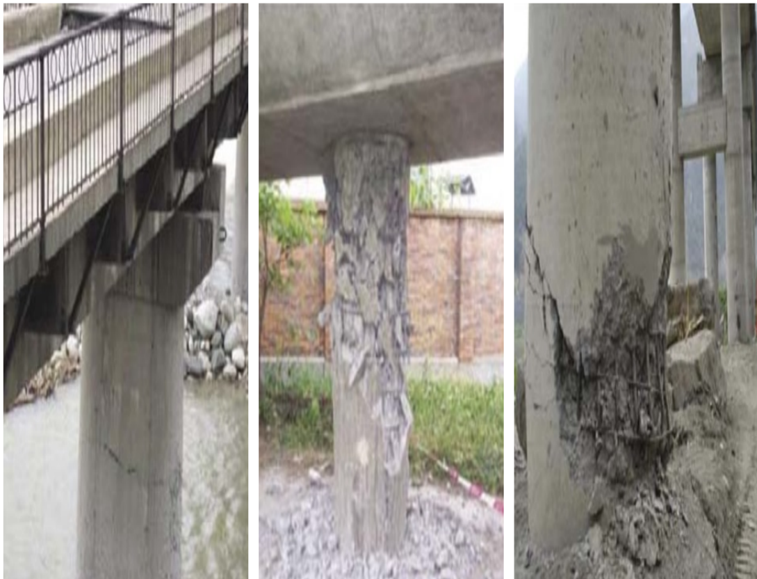
FIGURE 2.1: Bridge Pier Failures
