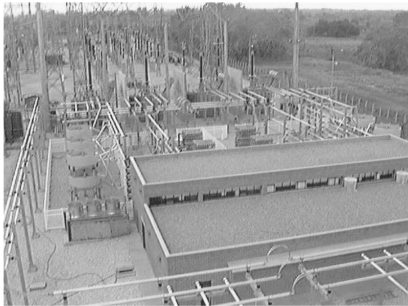
FIGURE 5.28 500 kV, 400 MVar SVC Chinu, I.S.A., Colombia. (Photo courtesy Siemens.)
