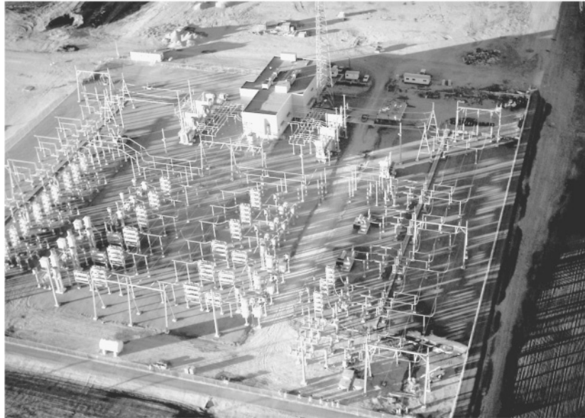
FIGURE 5.23 200 MW HVDC back-to-back converter station, at Sidney, Nebraska. (Photo courtesy Siemens.)
