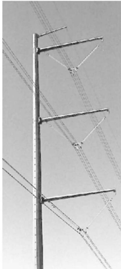
FIGURE 4.21 A 500-kV suspension tower with V string insulators.
