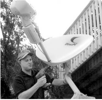
Figure 1-8 A satellite dish provides a 44,000-mile road to the global web. Photo by Advanced Network Services.
