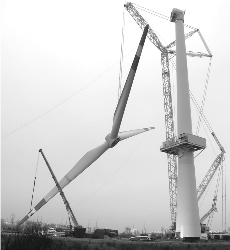
Fig. 15-13 Hoisting the Rotor by means of main mobile crane and assisting mobile crane [9]
