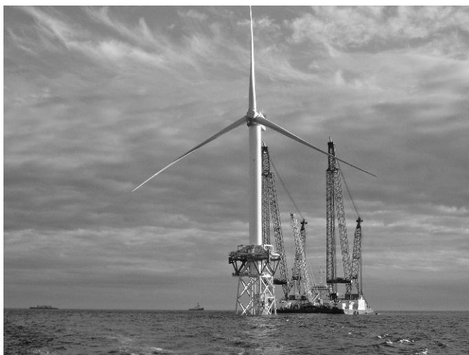
Fig. 16-9 Rotor installation at the Utgrunden wind farm with two jack-up barges and two tug boats [Photo Uffe Kongsted]
