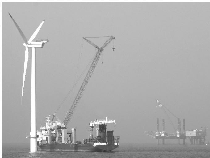
Fig. 16-8 Installation of an offshore wind turbine on a jacket support structure in 45 m water depth [REpower Systems AG]
