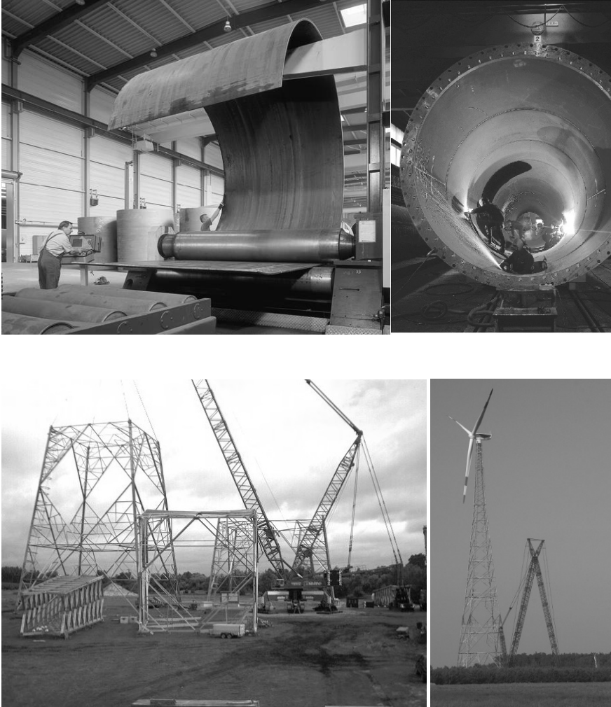
Fig. 3-53 Top: production of steel tube tower segments; left: bending of plate on 3-roll bending bench; right: welding together the plate of the tower segment (BWE); Bottom: FL 2500 in Laasow with 160 m lattice tower; left: assembling of the bottom tower segments; right: complete assembled wind turbine (Seeba, W2E, Fuhrländer)
