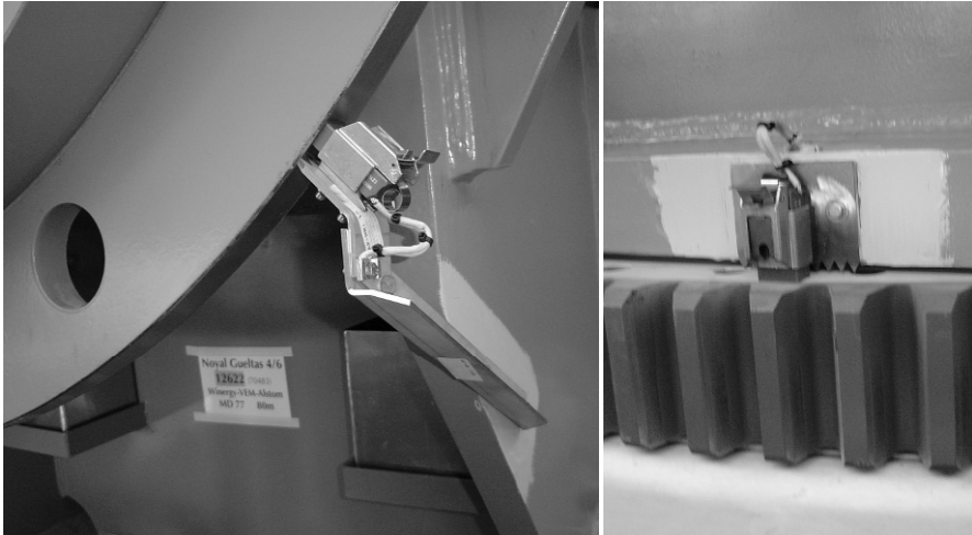
Fig. 3-47 Components of the lightning protection system for the protection of the bearings; left: sliding brush contact on the main shaft, right: on the yaw drive, combined with spark gaps (RE-power)
