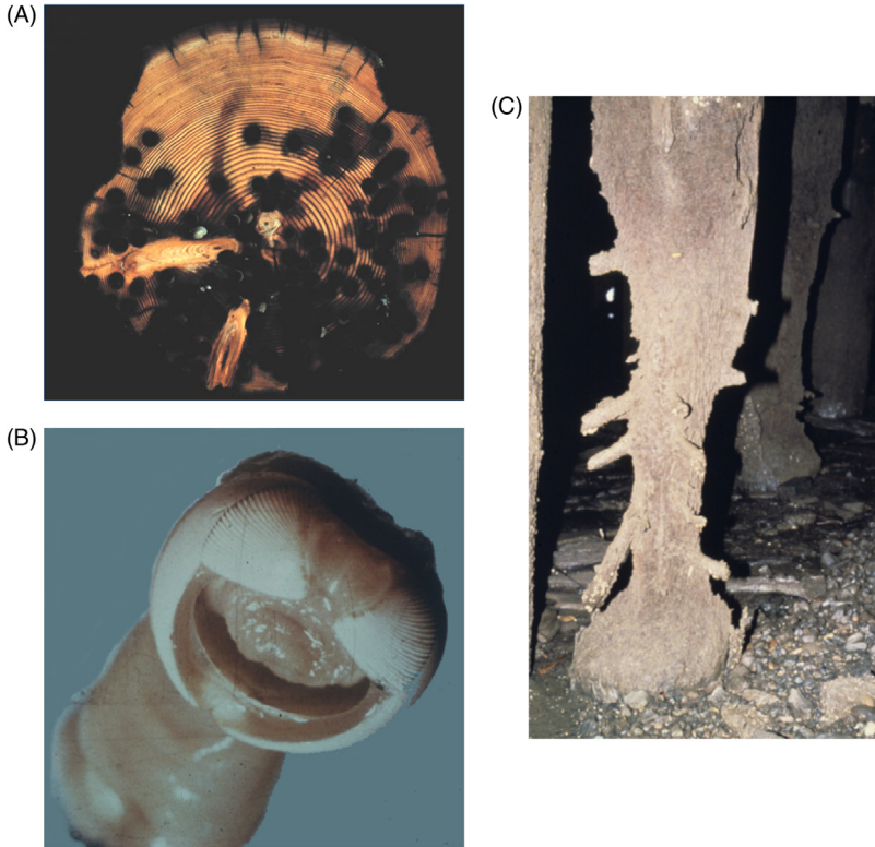
Figure 2.6 Marine borers cause severe damage to wood in salt-water exposures in some regions. (A) Cross section of a Douglas-fir piling showing numerous tunnels caused by Toredos sp. (B) Mouth parts of a shipworm removed for the wood. (C) Piling from the intertidal zone showing the hour-glass shape produced by Limnoria attack.
