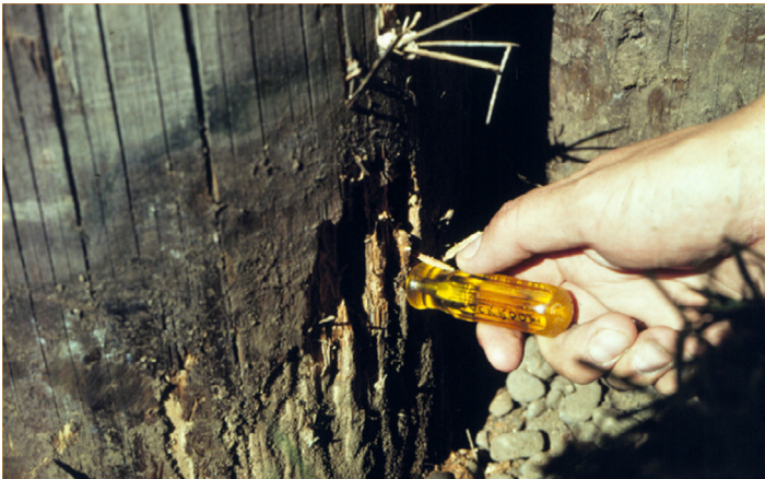
Figure 15.8 Typical soft rot damage in the groundline of a CCA treated Douglas-fir transmission pole that had been in service for approximately 10 years in a swampy area. Arrows (Left to right) identify the pole butt, zone of maximum soft rot development, and surface exfoliation and the groundline.
