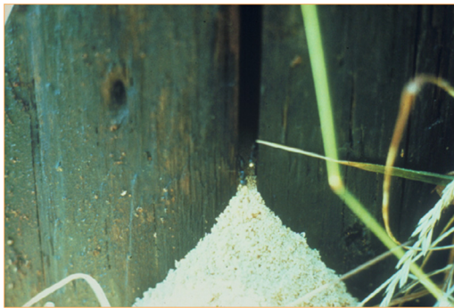
Figure 2.5 Carpenter ant invasion and internal damage in a treated Douglas-fir utility pole is indicated by the accumulating pile of fresh frass (arrow) at the base of the pole.
