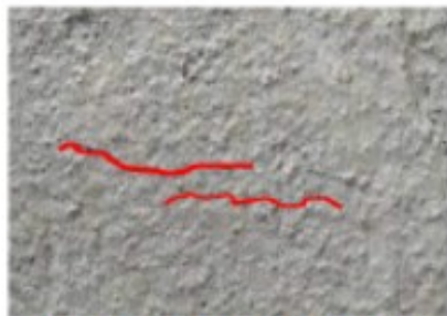
Early Age Micro-Cracking in Slab
