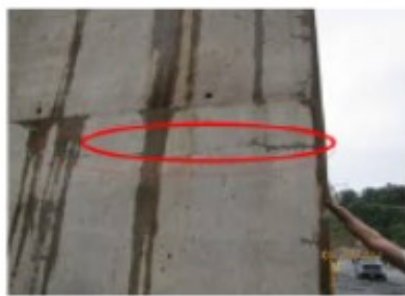
Cracks in compression
