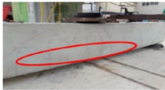
Cracks in beam
