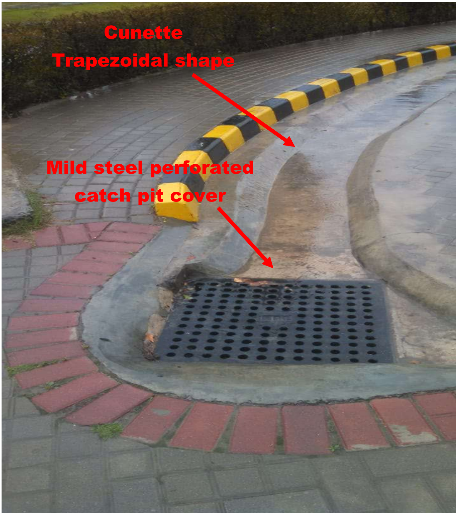
Fig P2: Photograph of Trapezoidal shape drain and perforated mild steel catchpit cover used for both systems
